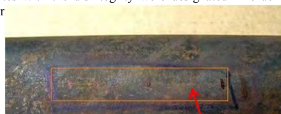
The disintegrity on the surface
